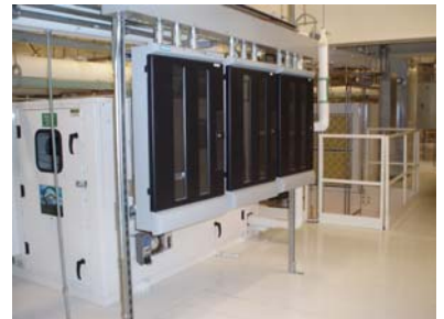
Building Automation System and Recirculating Air Handling Units, July 2007
